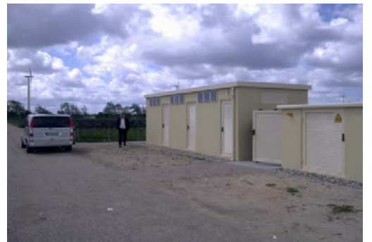
No. 4 View of Inverter & Transformer Buildings (Note the size relative to the vehicle)
